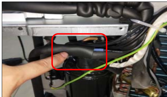
⑥Return air pipe temperature sensor
